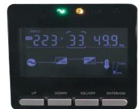
Panel de Control
